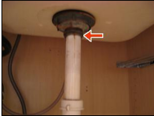
4.0 Picture 1 Right sink basin
