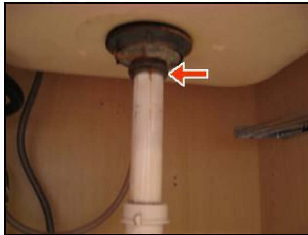
4.0 Picture 1 Right sink basin
